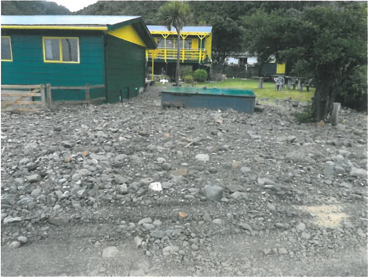
Material which has overtopped the seawall during the high seas
